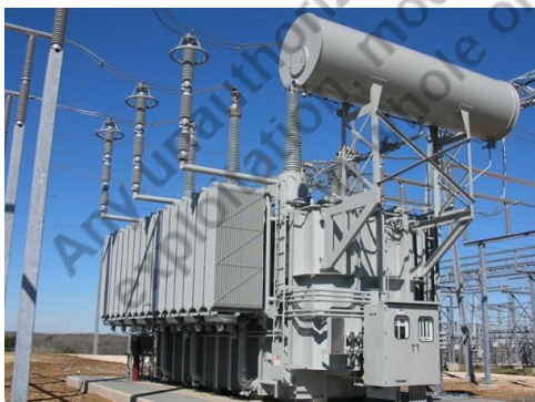
(a) Power Transformer
