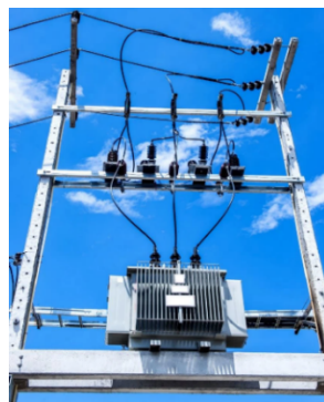
(b) Pole-mounted Distribution Transformer
